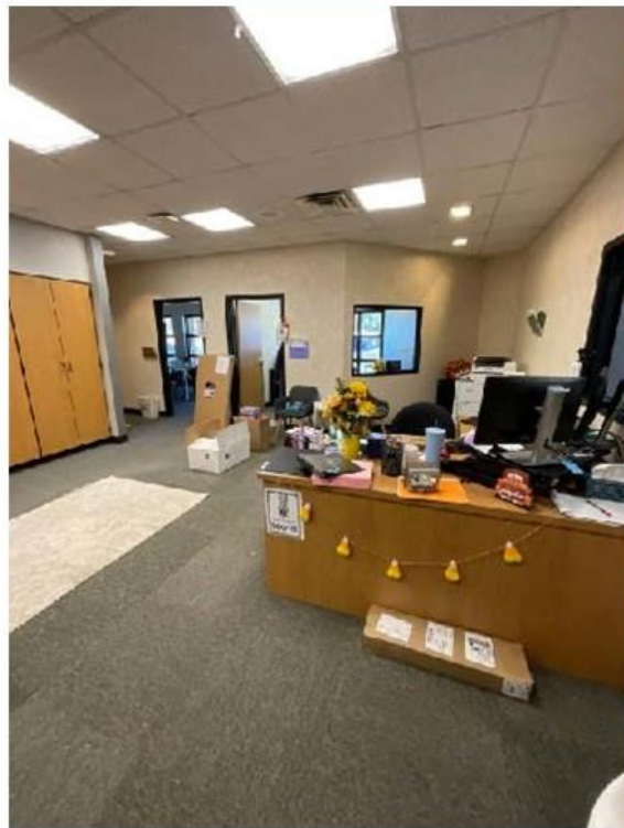
DOES NOT MEET TAS/ADA
