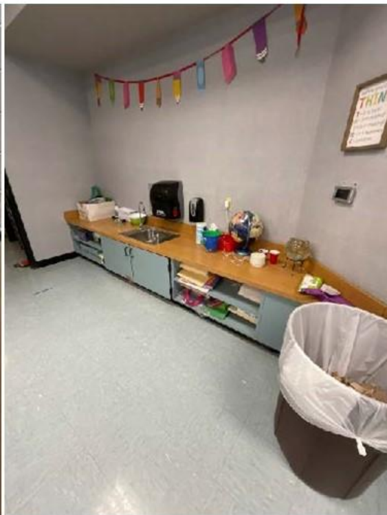
DOES NOT MEET TAS/ADA
