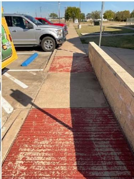
ADA RAMPS NEEDS REPAINTING
