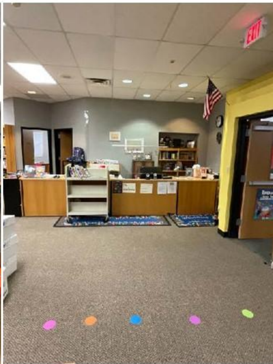
DOES NOT MEET TAS/ADA
