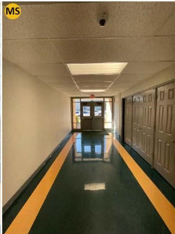
NEEDS SECURE VESTIBULE
