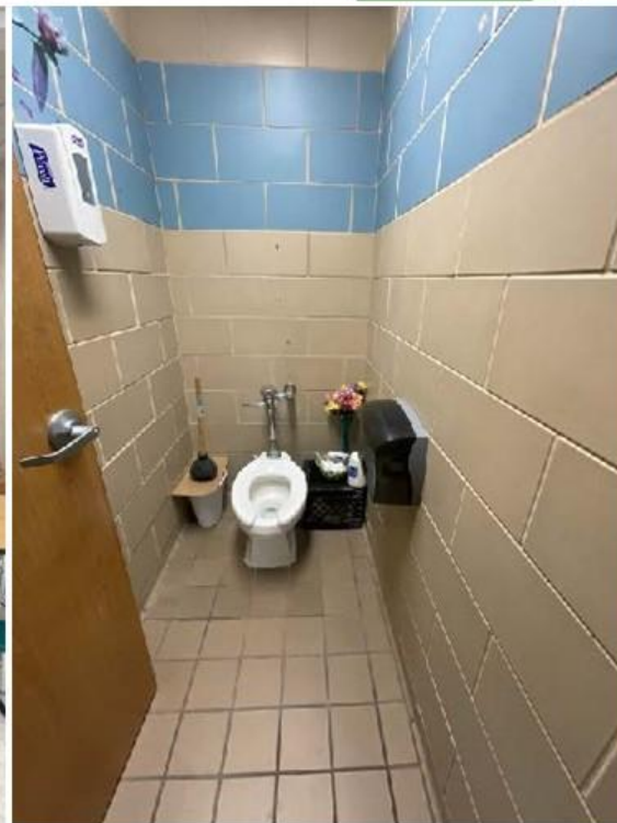
DOES NOT MEET TAS/ADA
