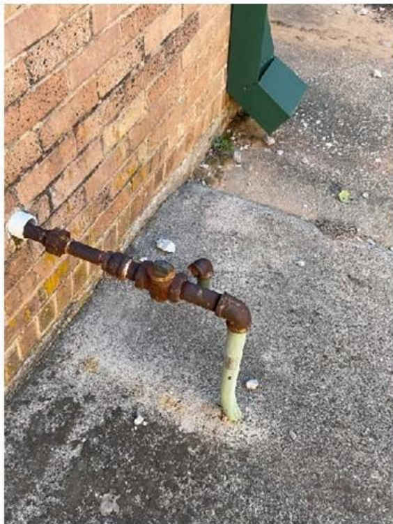
SAFETY RISK / GAS LINE NEEDS REPAINTED
