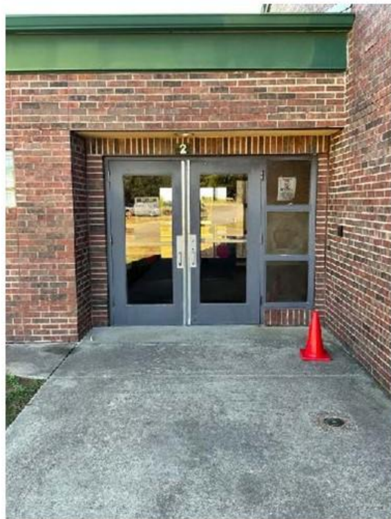
NEEDS SECURE VESTIBULE
