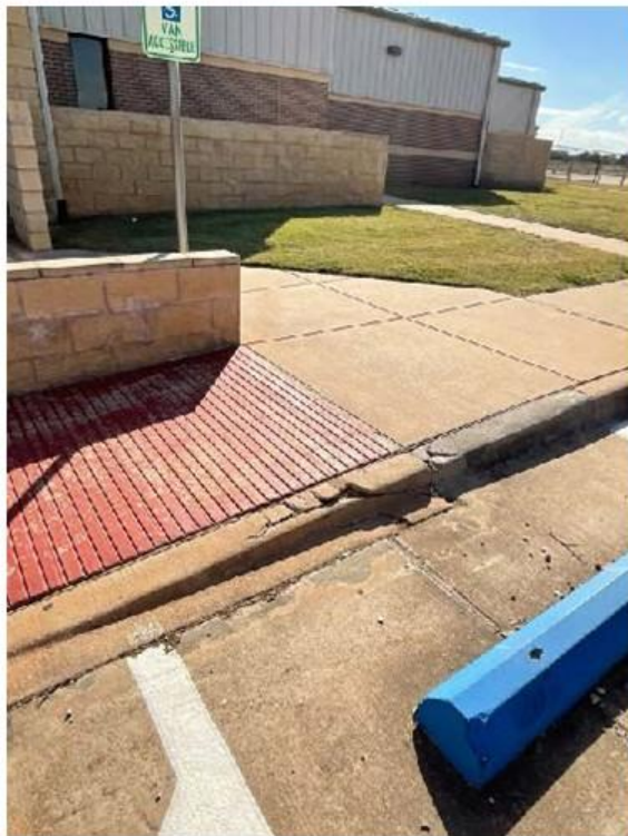
ADA RAMPS NEEDS REPAINTING
