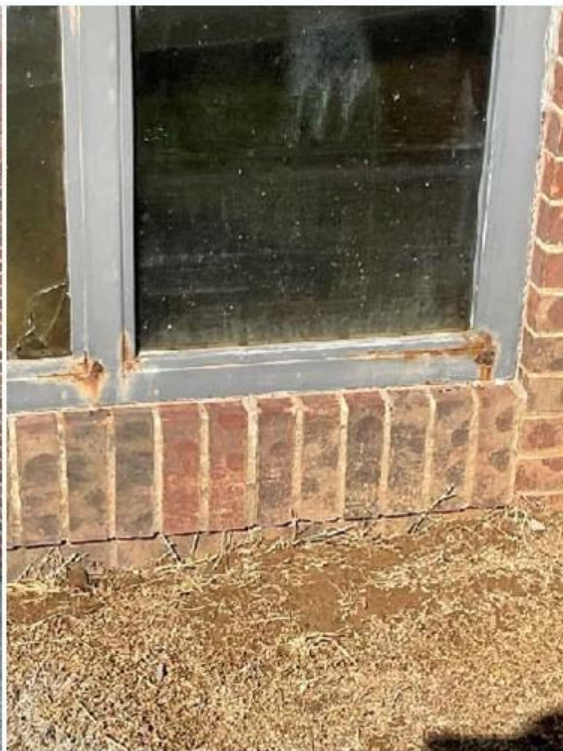
DETERIORATING WINDOW FRAME
