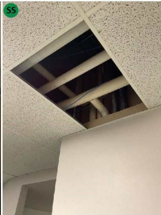
MISSING CEILING TILE
