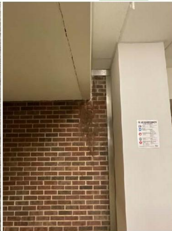
EVIDENCE OF MOISTURE
