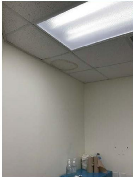
EVIDENCE OF MOISTURE DAMAGE
