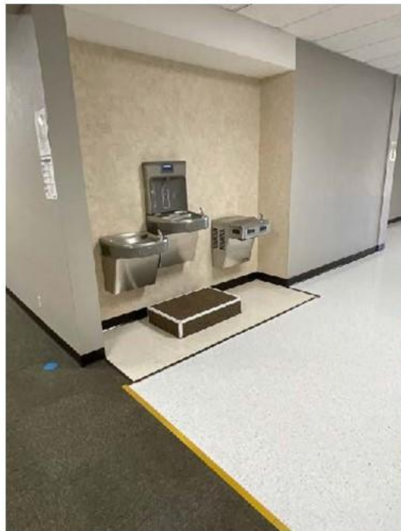
DOES NOT MEET TAS/ADA
