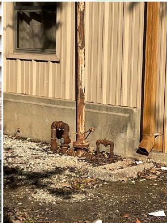
SAFETY RISK / UTILITY LINES NEED REPAINTED
