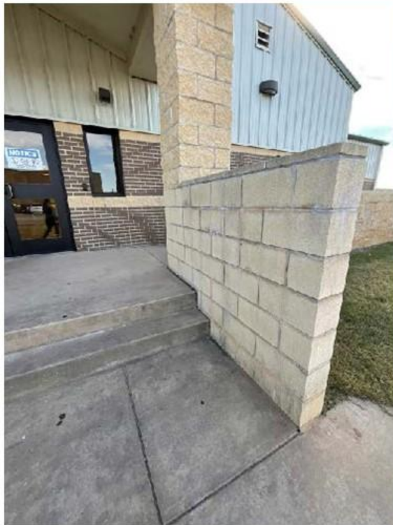
HANDRAIL MISSING / SAFETY RISK
