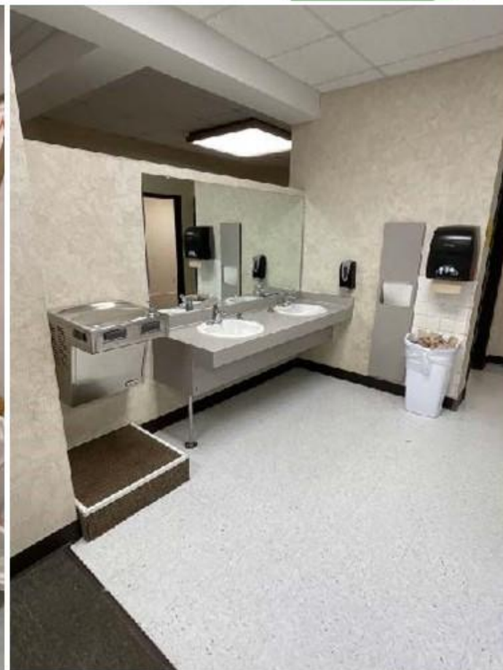
DOES NOT MEET TAS/ADA
