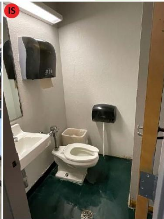
DOES NOT MEET TAS/ADA
