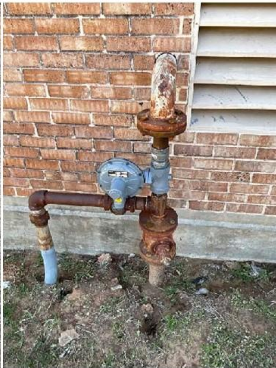
SAFETY RISK / UTILITY LINES NEED REPAINTED
