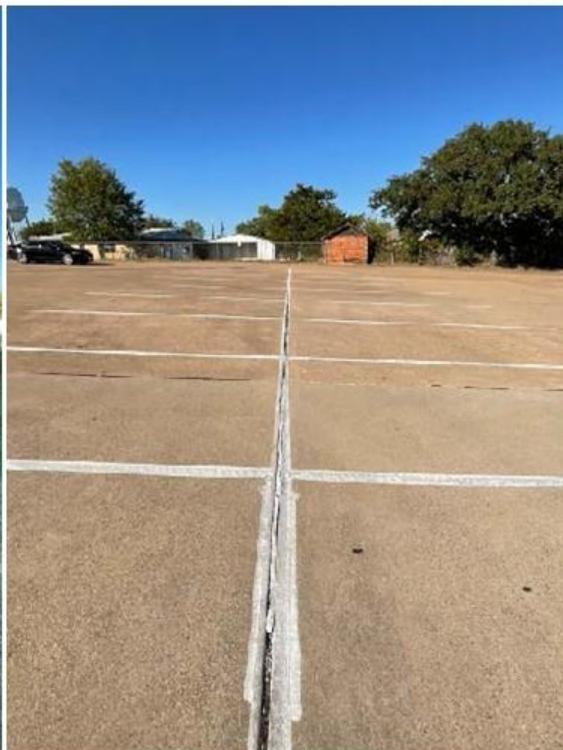
PAVEMENT STRIPING FADING
