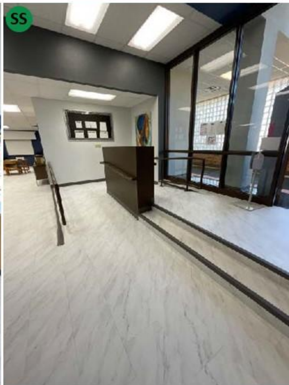
DOES NOT MEET TAS/ADA
