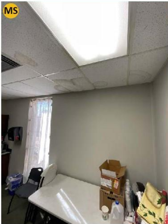
EVIDENCE OF MOISTURE DAMAGE
