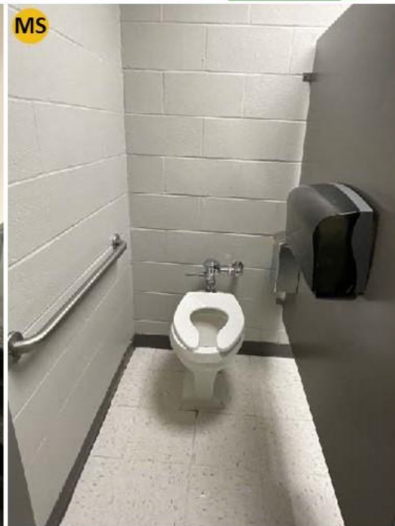
DOES NOT MEET TAS/ADA
