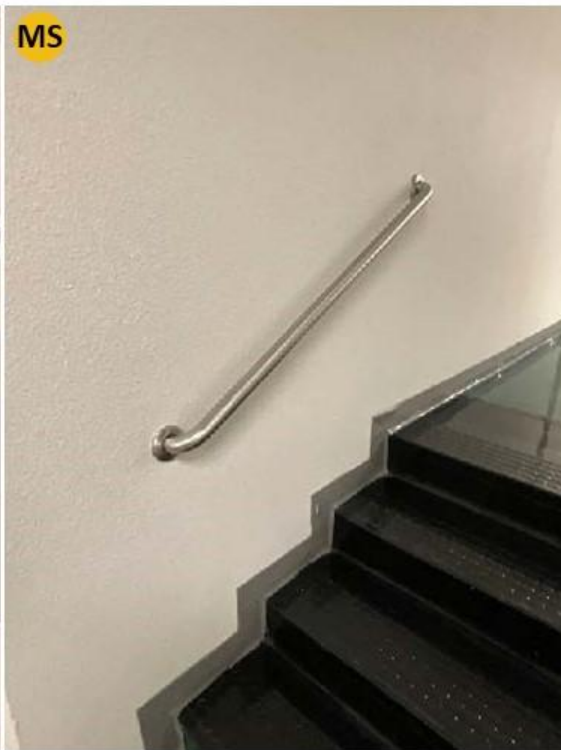
DOES NOT MEET TAS/ADA
