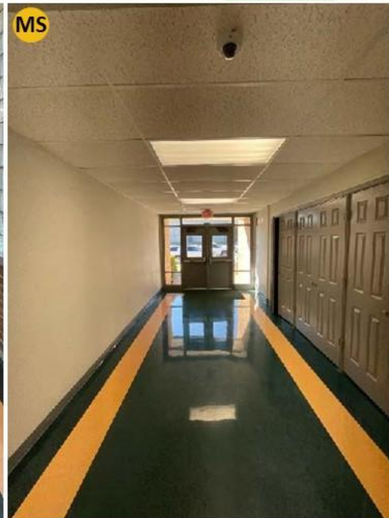
NEEDS SECURE VESTIBULE
