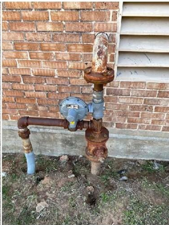
SAFETY RISK / UTILITY LINES NEED REPAINTED
