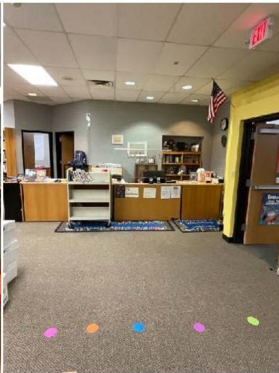
DOES NOT MEET TAS/ADA
