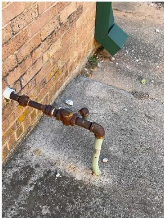
SAFETY RISK / GAS LINE NEEDS REPAINTED
