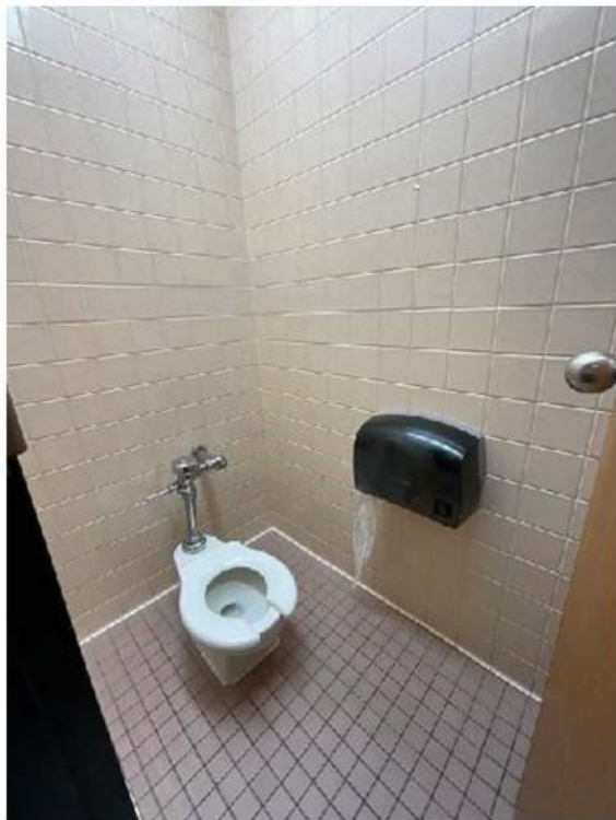
DOES NOT MEET TAS/ADA
