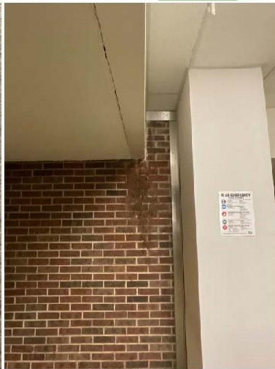
EVIDENCE OF MOISTURE
