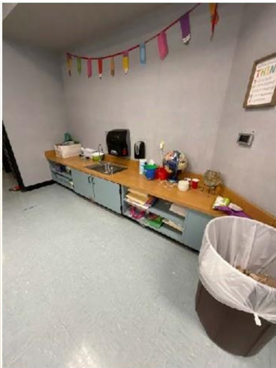
DOES NOT MEET TAS/ADA
