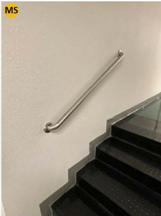
DOES NOT MEET TAS/ADA
