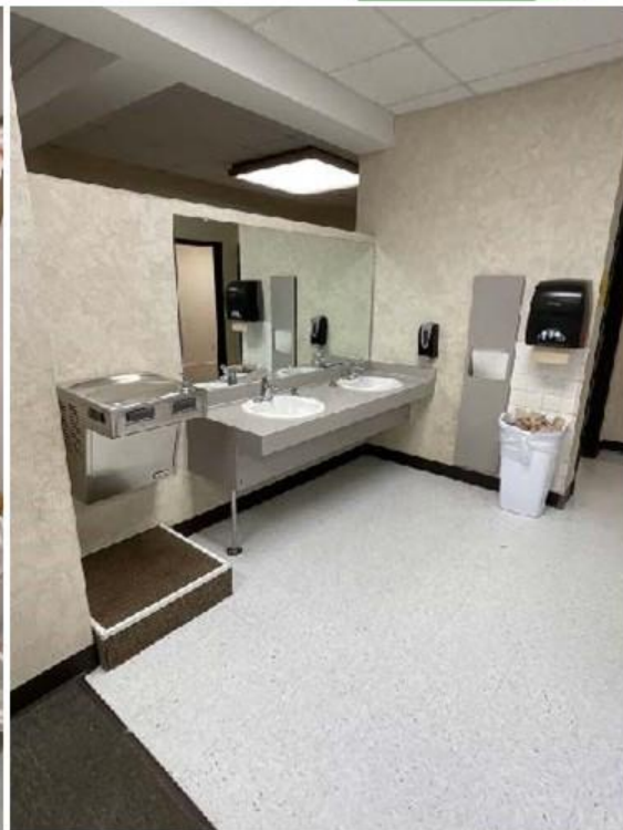
DOES NOT MEET TAS/ADA
