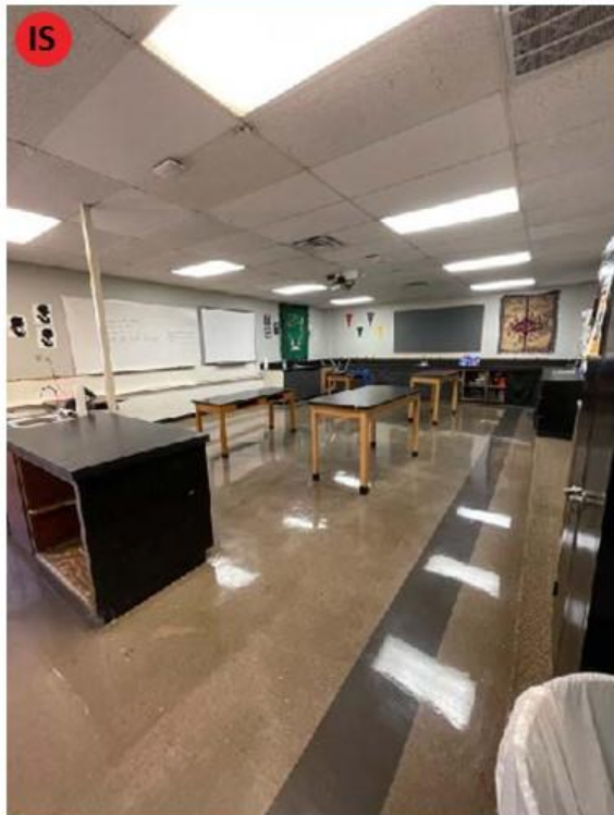
DOES NOT MEET TAS/ADA
