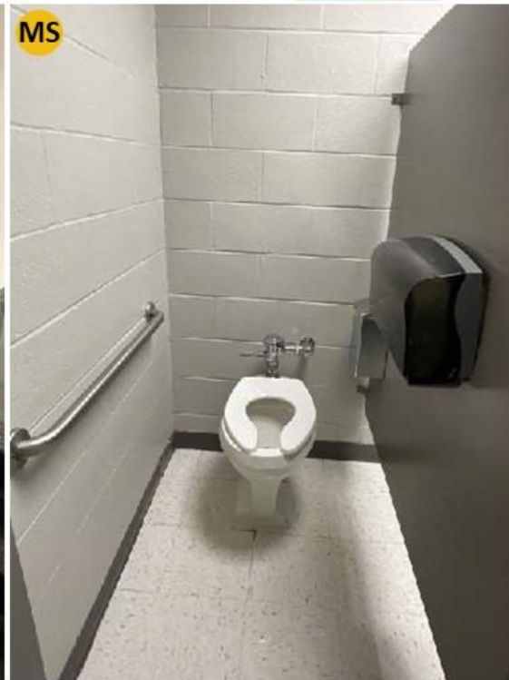
DOES NOT MEET TAS/ADA
