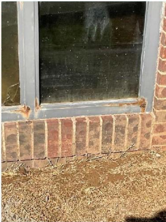
DETERIORATING WINDOW FRAME
