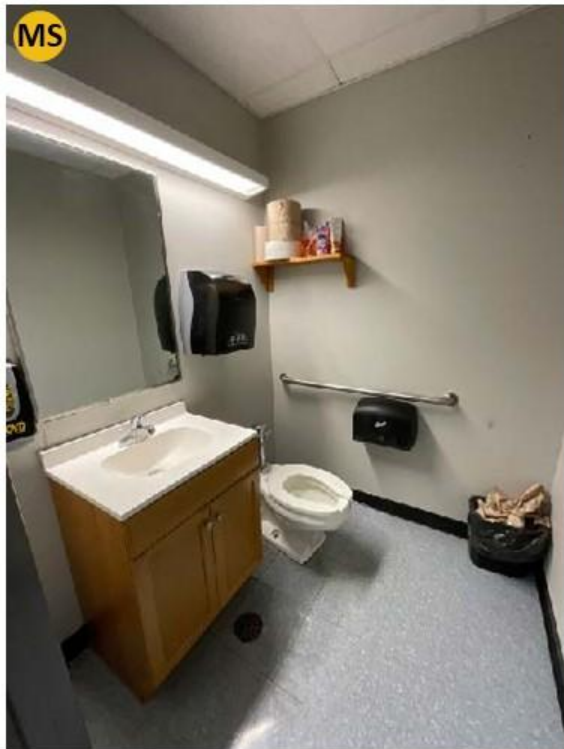
DOES NOT MEET TAS/ADA
