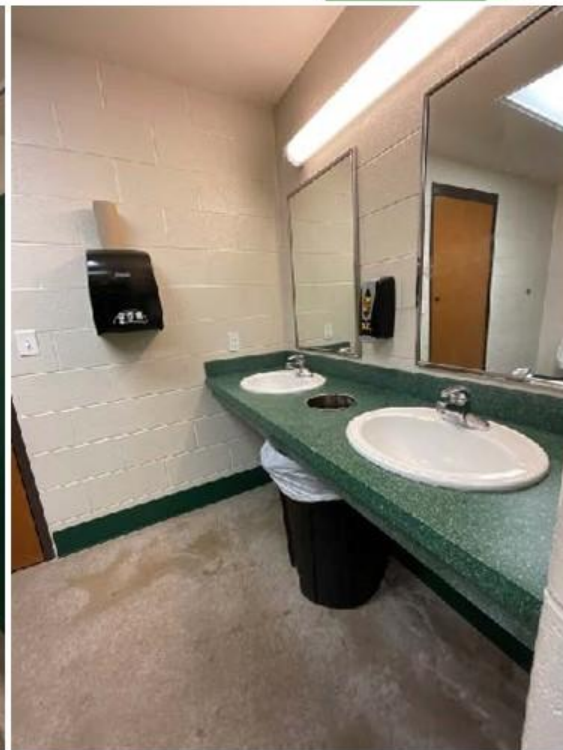
DOES NOT MEET TAS/ADA
