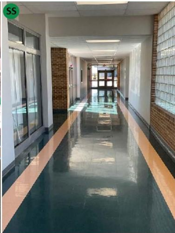
NEEDS SECURE VESTIBULE
