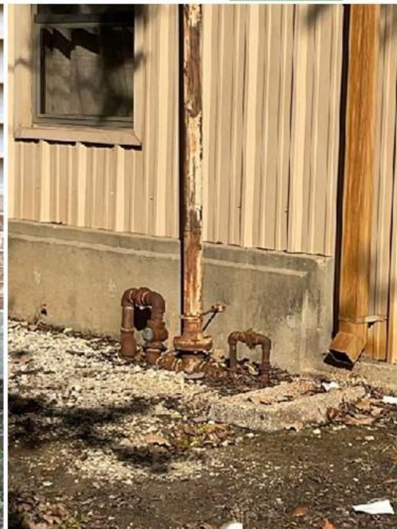
SAFETY RISK / UTILITY LINES NEED REPAINTED
