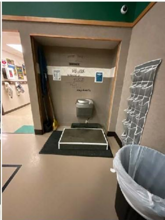
DOES NOT MEET TAS/ADA
