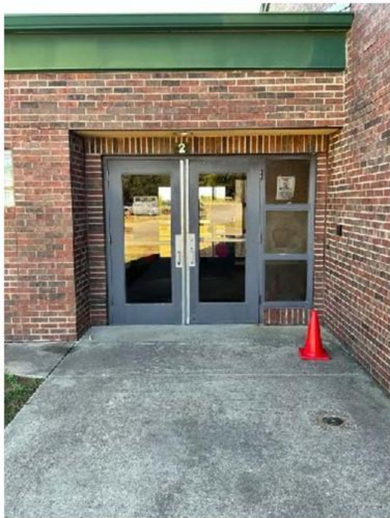
NEEDS SECURE VESTIBULE
