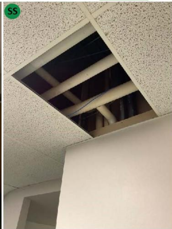
MISSING CEILING TILE
