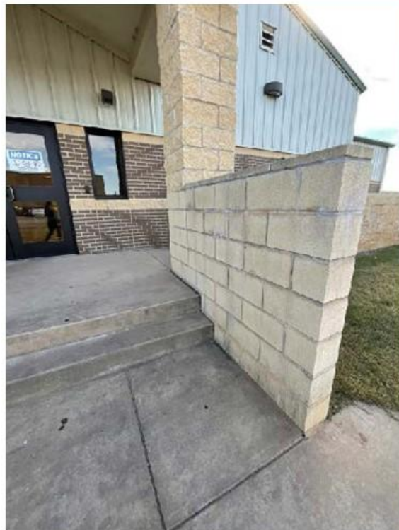
HANDRAIL MISSING / SAFETY RISK
