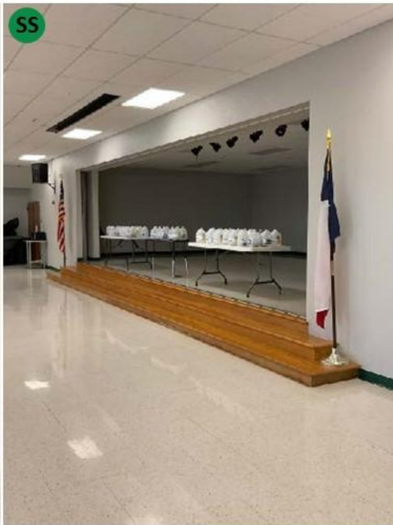
DOES NOT MEET TAS/ADA
