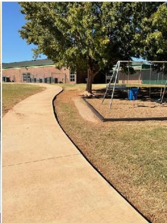
DOES NOT MEET TAS/ADA
