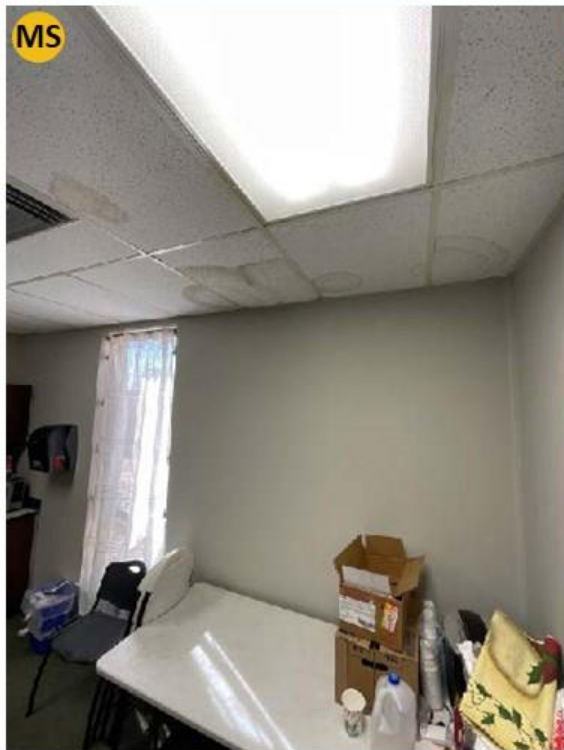
EVIDENCE OF MOISTURE DAMAGE
